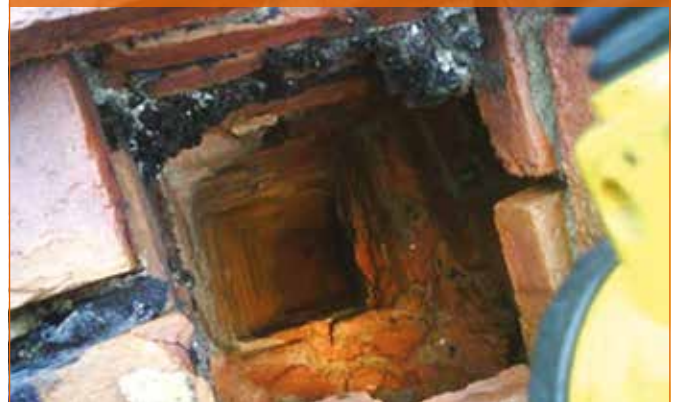
Image 1: Chimney in poor condition
